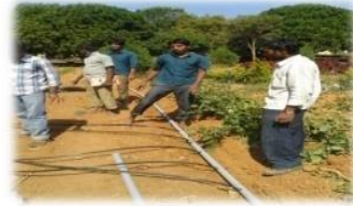
Lateral connection to Submain Pipes
